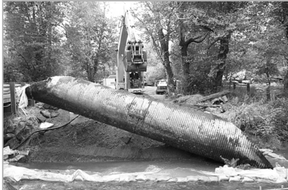
Removing culvert in Western Washington. Photo by So Puget Sound Salmon Enhancement Group
